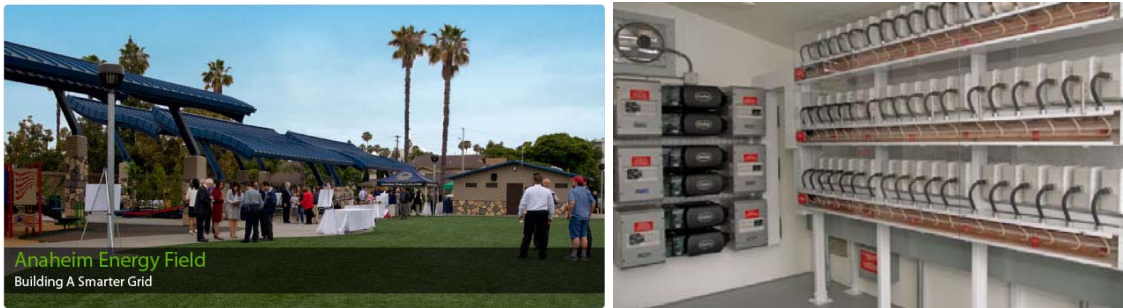
Photos of a Solar Energy Park with lithium ion battery storage
